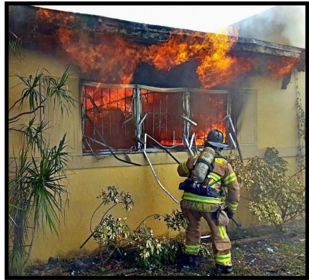
(FIGURE 8) FF CAMERO IS WORKING IN COORDINATION WITH THE ATTACK TEAM TO EFFECTIVELY VENT THE FIRE COMPARTMENT. AS WELL AS CLEARING OUT THE ENTIRE WINDOW, CREATING A SAFE SECONDARY MEANS OF EGRESS FOR THE INTERIOR FIREFIGHTERS.
